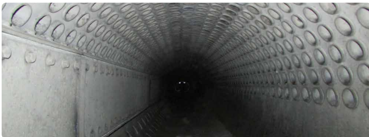
Blue Reef Water Solutions: High-pressure boiler mud drum free of scale after treatment with Blue Reef products.
